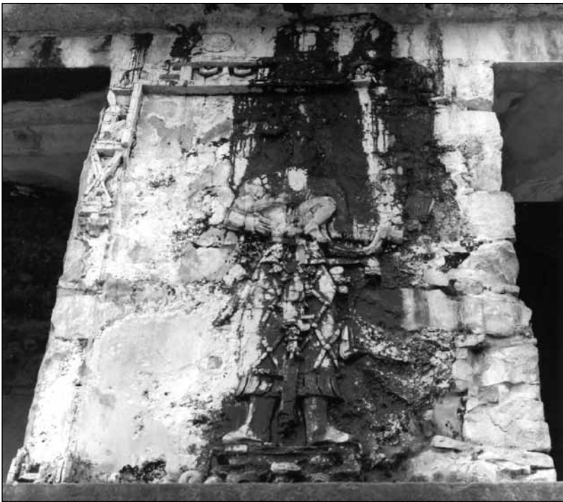
Acid rain impact on Temple of the Inscriptions pier
