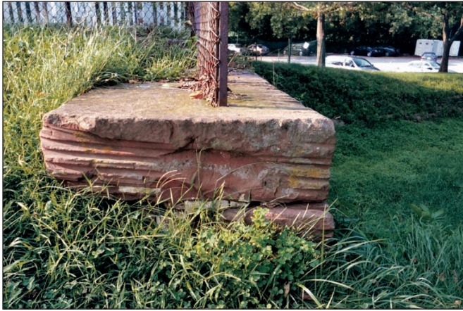
Figure 4. Rope grooves on downstream corner of Rileys Lock #24, Maryland (photo by Ron Canter).
